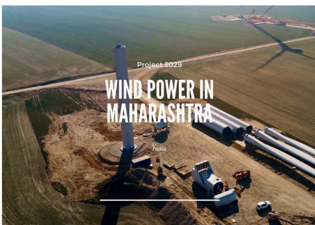
Project 3029: Wind Power in Maharashtra
